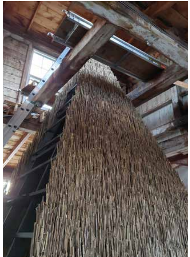
Images: (Left) Construction of The Hissing Folly , (above) thatching of The Hissing Folly , photos by Harry Knight, 2020.
